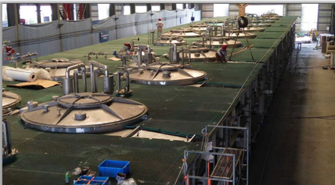
Solvent Extraction Plant Factory Acceptance Test
