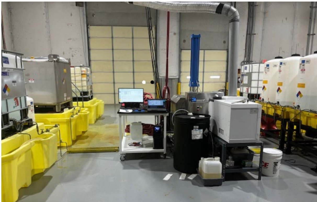
Figure 1: Rare Earth Technologies (RETi) 3 Mt/y pilot separation facility in USA
