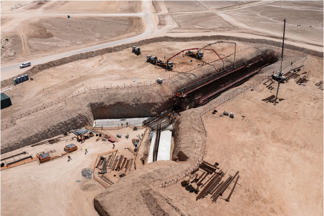
Figure 3: With the stockpile tunnel foundation completed, focus now shifts to the tunnel and wing walls.
