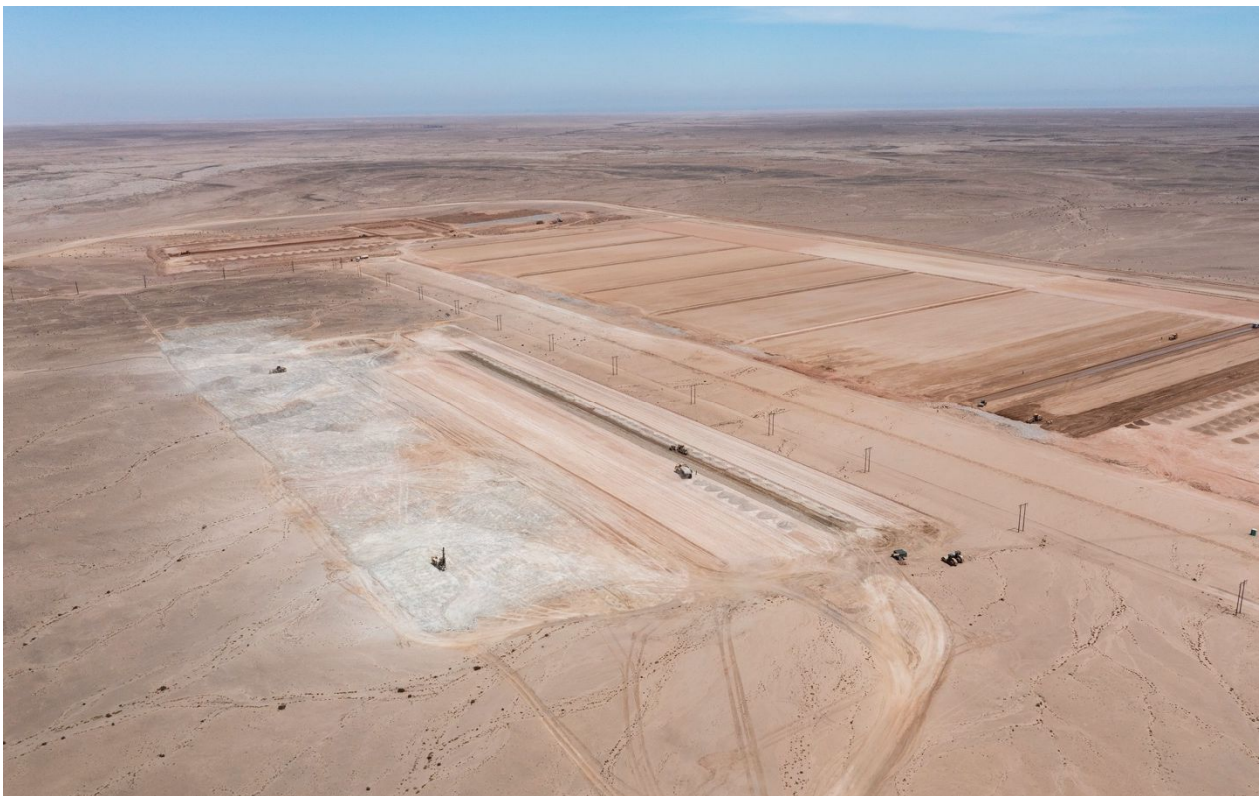
Figure 1: In addition to the heap leach pad earthworks, works have now begun on the wet plant terraces.
