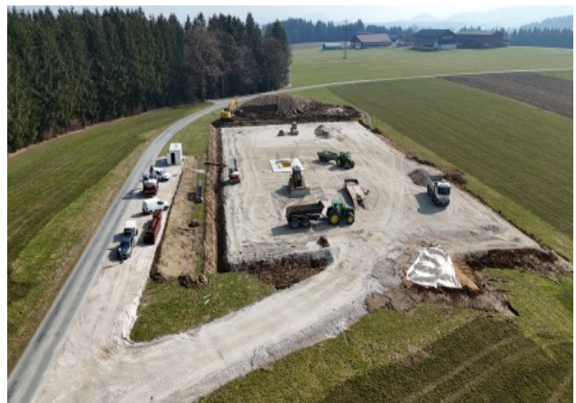
HOCH-1 rig site construction in the ADX-AT-I Licence during February 2026 in preparation for the commencement of drilling in April 2026
