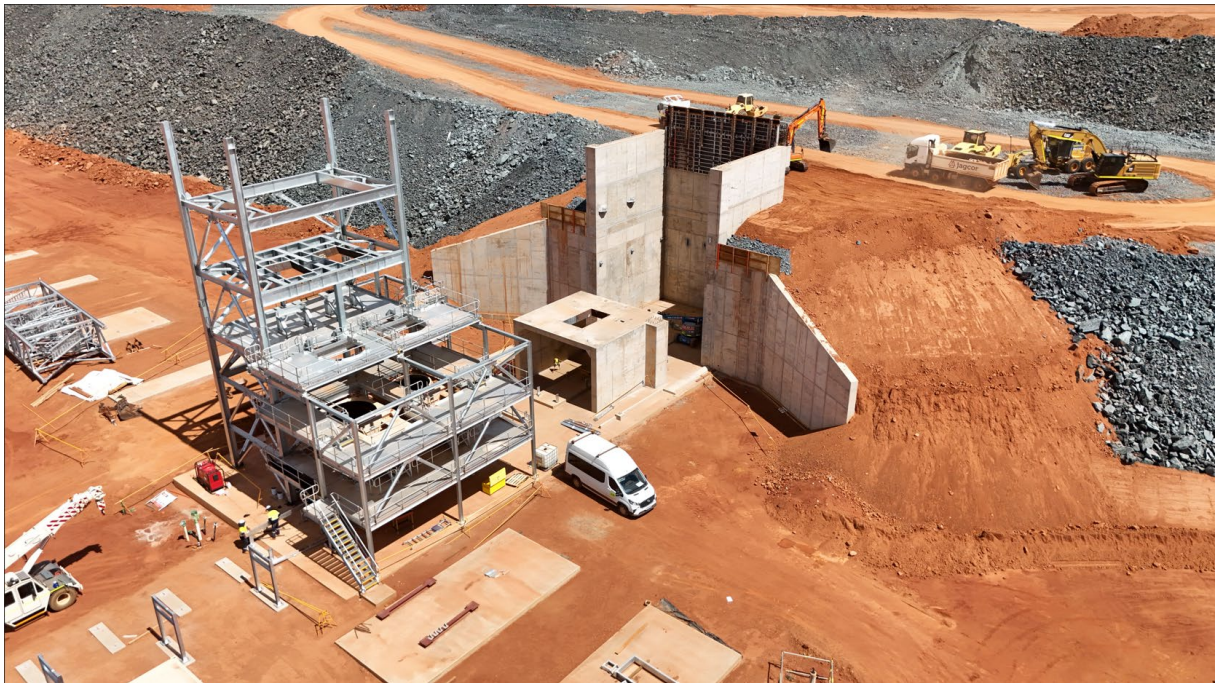
Primary/Secondary/Tertiary crusher building and ROM 2 tie in.
