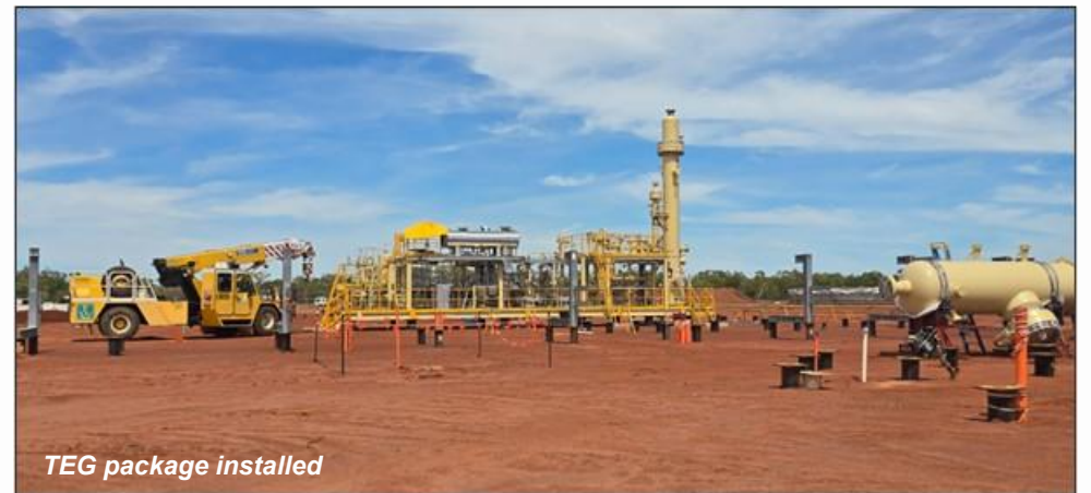
Compressor units installed on SS2 pad
