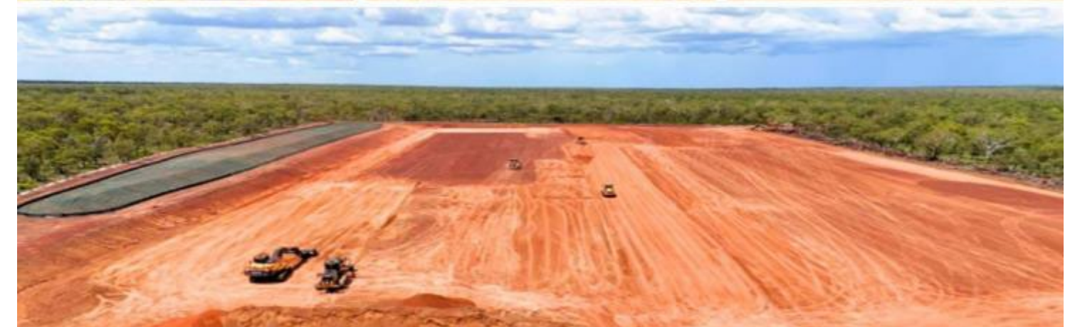
Early works for the Carpentaria Gas Plant including clearing, earthworks and refurbishment of equipment in Roma commenced in early October 2025
