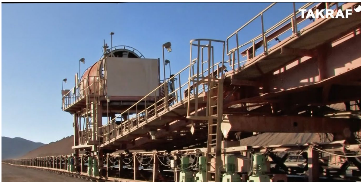
Image 1: Long conveying systems designed and installed by Takraf (Source: Takraf)
